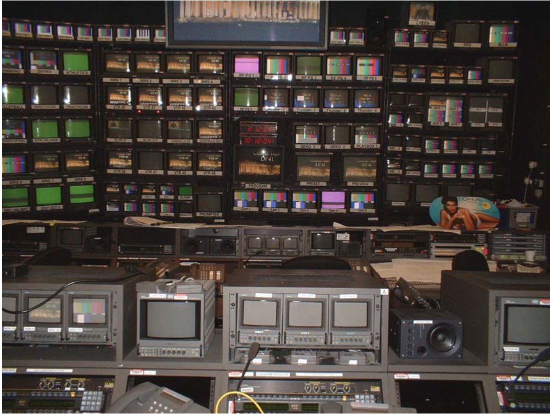
The NBC® broadcast control room – RTS® keypanels in foreground
