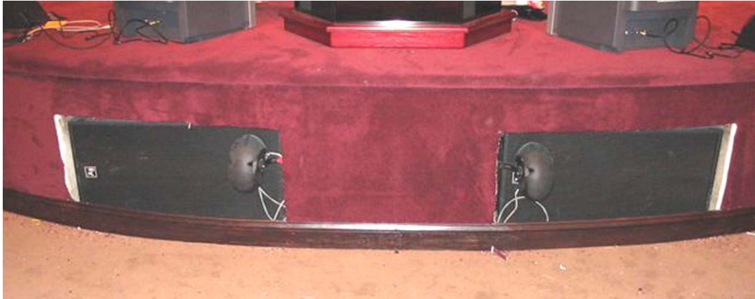
QRx subs embedded under the stage, sans covering. See prior photo for finished effect.
