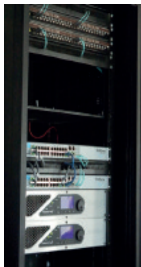
Nion3 processors in the rack
