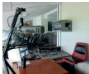
The simple control room at Loftus Versfeld
