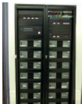
One of the amp racks at Loftus Versfeld
