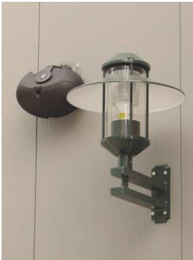
One of 164 EVIDs Installed Throughout the Stadium
