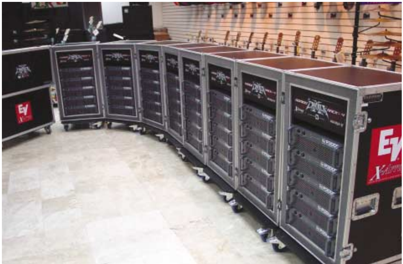
La Changa's Custom Racks: Loaded with EV P3000 Power Amps
