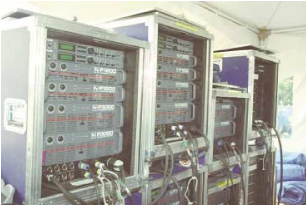
Racks of EV Precision Series Amplifiers
